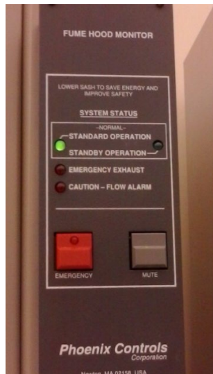
Figure 3. MLSC hood Phoenix Controls unit indicating proper operation. Note green light lit.
