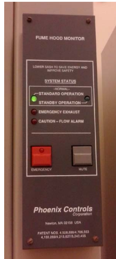
Figure 3. MLSC hood Phoenix Controls unit indicating proper operation. Note green light lit.
