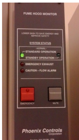
Figure 3. MLSC hood Phoenix Controls unit indicating proper operation. Note green light lit.
